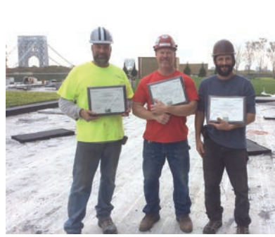
Dave Sondermeyer, Mike Leonard & Rich Quayle at 100 Park in Fort Lee, NJ. All three of our trades are working on The Modern's 2nd Tower, another 47 story luxury high-rise at the foot of the George Washington Bridge.
