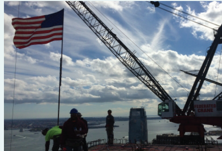
"Our plumbers are setting roof drains and sanitary vent sleeves at a project in Jersey City, NJ." - Mike Buttermark , Plumbing Project Manager
