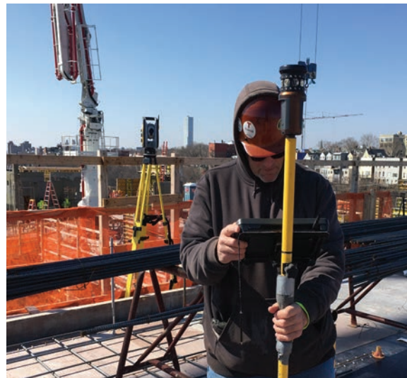
Pictured Above: Hank Bell using the Robotic Total Station at 700 Jackson in Hoboken, NJ. All three of our trades are working on this site.
